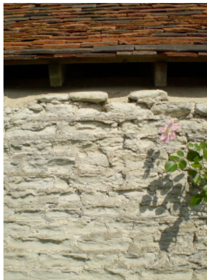
The wall of a barn in Mackney, - built of chalk clunch which has become soft and flakey over the centuries.
