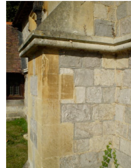
St James' church: walls of hard sandstone blocks with corner stones of shaped Jurassic limestone
